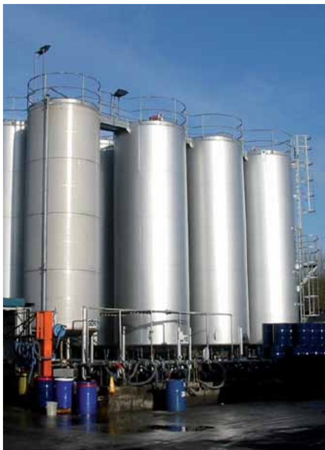
Multisol's Tank Farm
